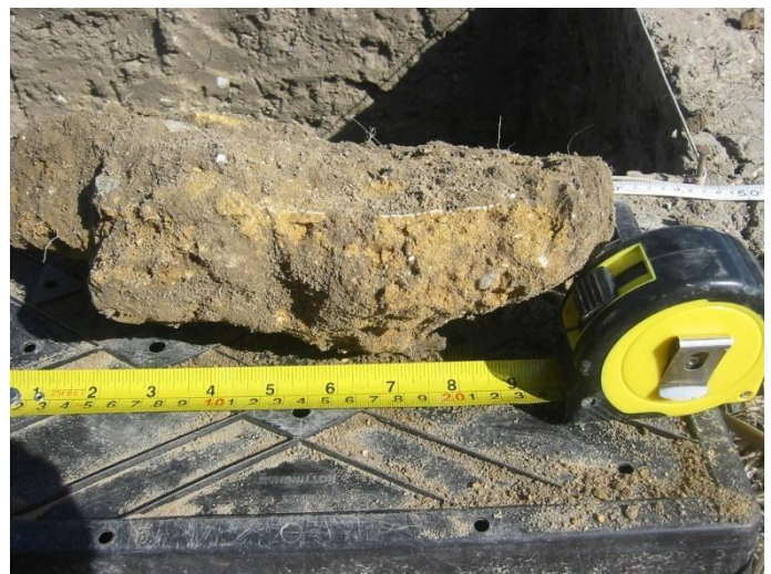
Figure 23 - Large chunk of mortar extracted from side of trench B The thin white line of plaster can be seen uppermost
